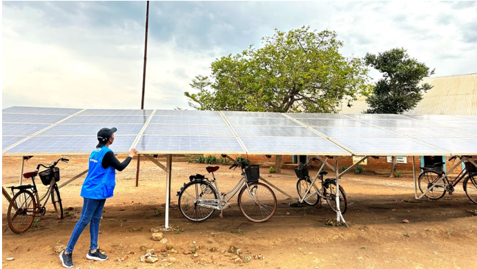
Solar PV system installed at Multipurpose Community Centre in Nyarugusu Refugee Camp in Tanzania. Photo: UNHCR Tanzania
